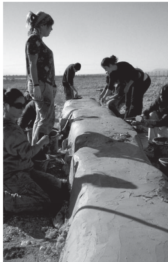
Students at Courtney Rosser’s course apply a second coat of mud plaster to a bench they built using tires and trash as the structure.
